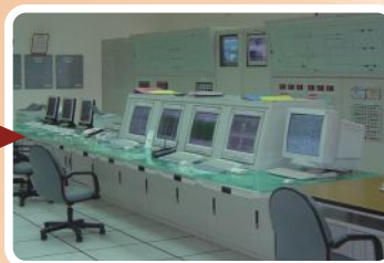
Disaster Prevention Centre (Control room).
