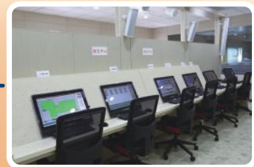
YunYang remote monitoring center (Control through network connection).
